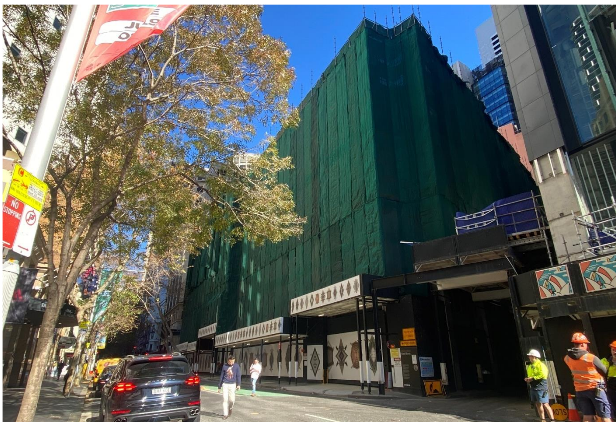
Figure 2: Existing site under demolition viewed from Pitt Street with existing gantry hoarding (servicing construction site to the north) along Underwood Street
